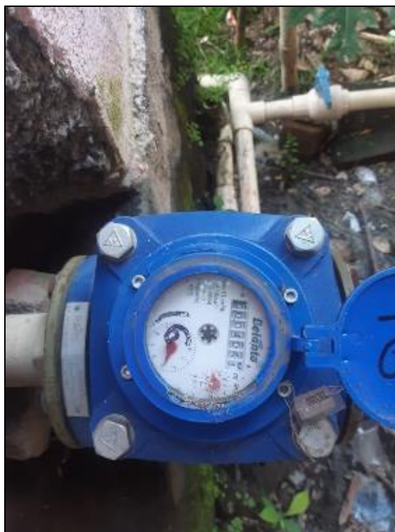
Figure 4-20: Sample photo of flow meter
