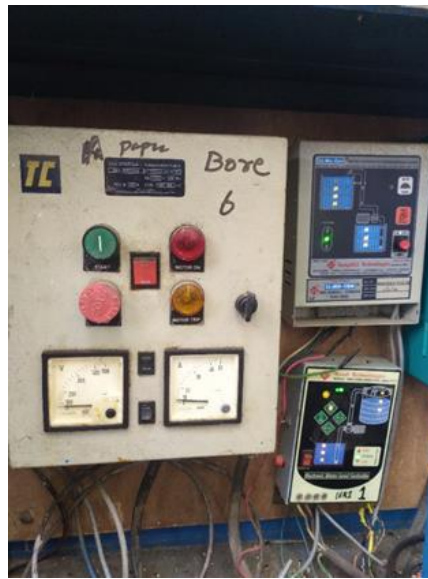
Figure 4-4: Bore-well pump panel and level controller switch
