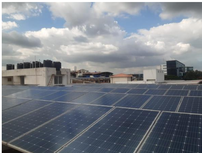
Figure 5-14: Sample photo – SRTPV system
