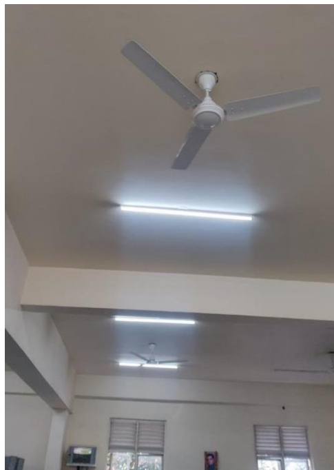
Figure 5-13: LED lights in Classrooms, Labs, and Corridors
