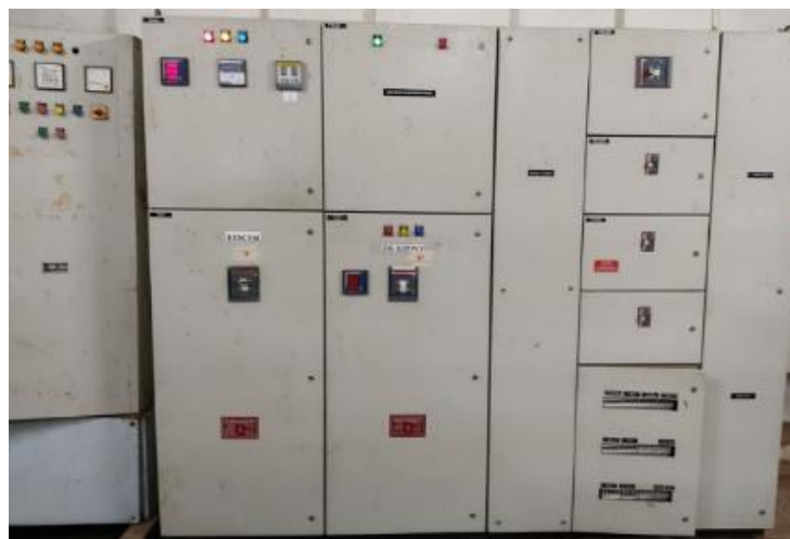
Figure 5-2: Electrical Panel Room
