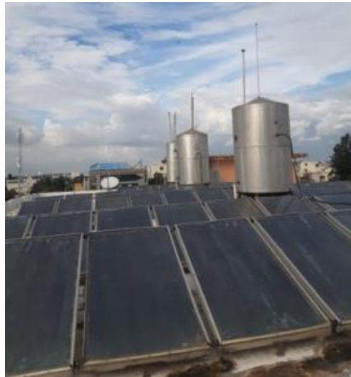
Figure 4-13: Hot water system in hostel
