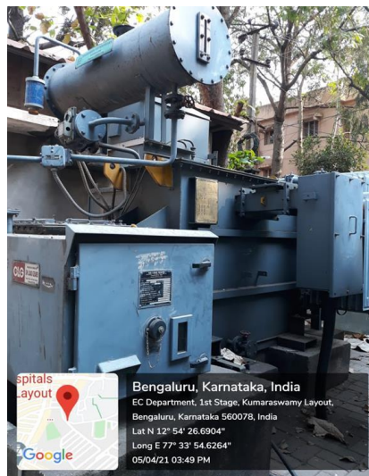
Figure 5-1: Transformer unit Installed in the campus
