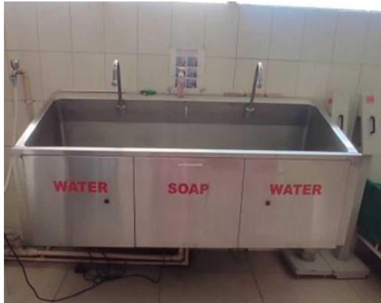
Figure 4-19: Sensors based wash basin
