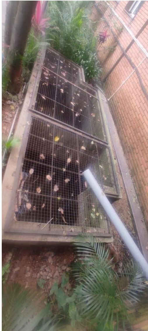
Figure 4-11: RWH sump near dental blocks
