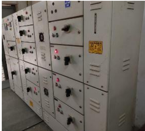
Figure 5-3: Capacitor Bank Panel
