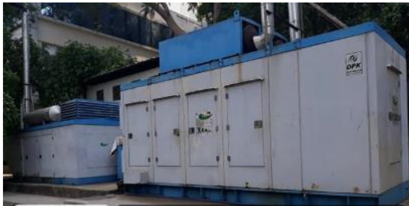
Figure 5-4: 400kVA and 250 kVA Diesel Generator (DG) set
